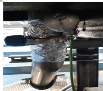
Discharge Temp Measurement
