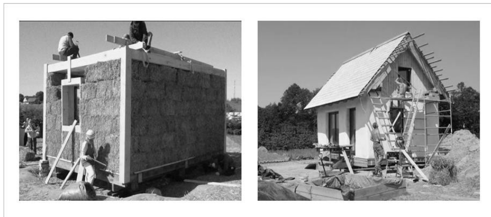
Figure 5.14. Prototype of open-source house 'Nano-habitat' during a) wall construction, b) plastering. Photo courtesy of Paweł Sroczyński 157
