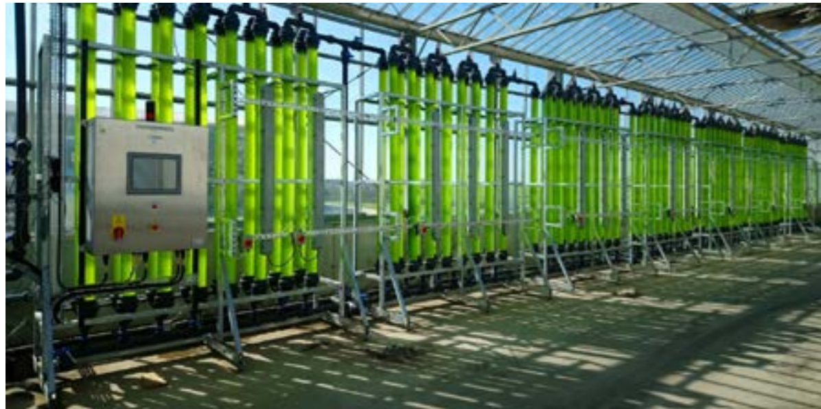
Figure 4: 7 tonnes photobioreactor installed at the Langage AD site. Image shows the light phase of the facility (i.e. vertical tubes) and the control panel allowing for parameter control and monitoring.
