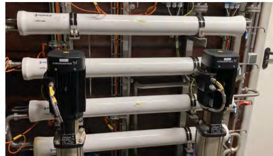
Reverse osmosis membranes
