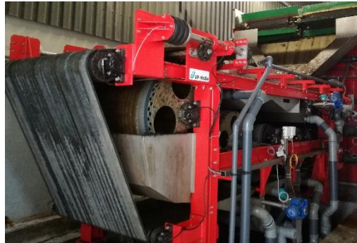
Figure 2-8 Belt press. Source: VP-Hobe, installed at BioStorg Biogas Plant, Houthalen-Helchteren, Belgium, 2019.
